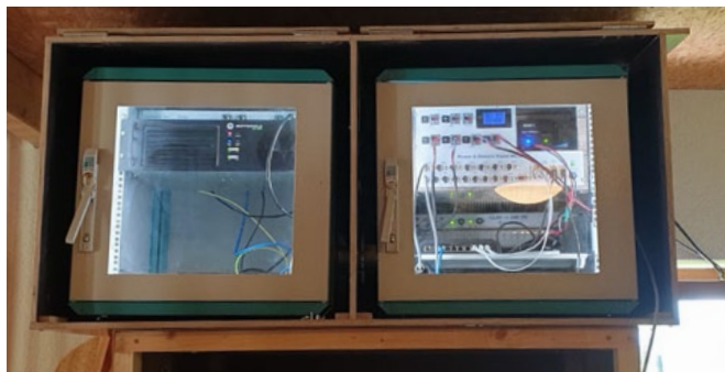
Linkes Rack: DMR Repeater Motorola DR3000
